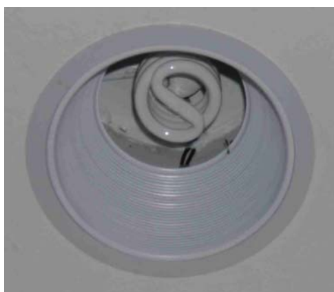
Figure 13. White painted reflector with 23 watt spiral CFL
