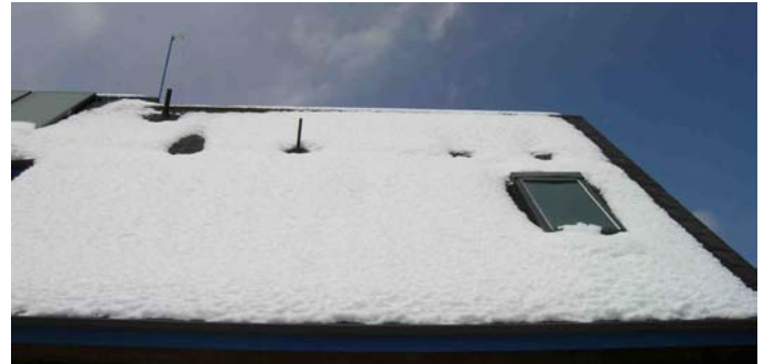
Figure 7. The two holes in the snow above the skylight correspond to recessed can lights in a bedroom that are almost never turned on. Melting is due only to air exfiltration from the conditioned space below the cans and the lack of insulation on top of them. The larger melted hole in the snow to the left of the vent pipe is due to a similar can above the shower which has a 250 watt infrared bulb in it. This light is on a timer and on average is illuminated about 12 minutes a day.
