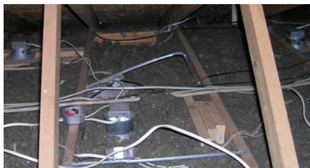
Figure 15. Leaky cans crisscrossing poorly-insulated attic
