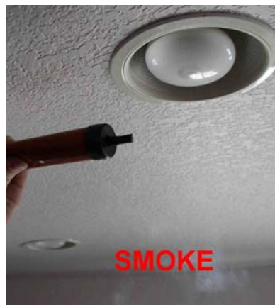
Figure 4. Can light in a kitchen ceiling with a blower door depressurizing the home. Smoke indicates openings to the vented attic above.
