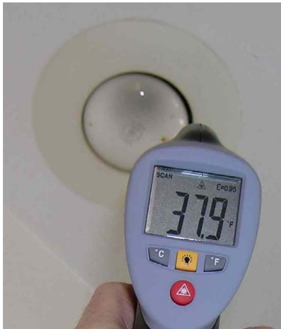
Figure 6. Kitchen light in a home heated to 68°F, outside air temperature of 34°F, blower door depressurizing the home
